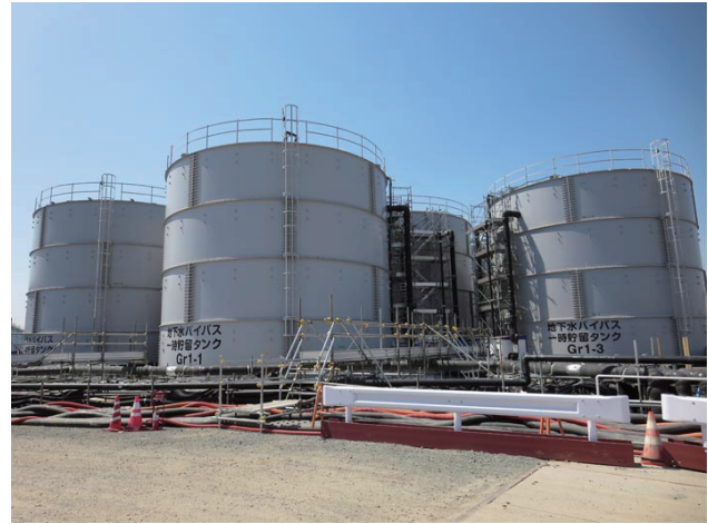
Ground water storage tanks at Fukushima Daiichi Nuclear Power Station (Photo by TEPCO)
