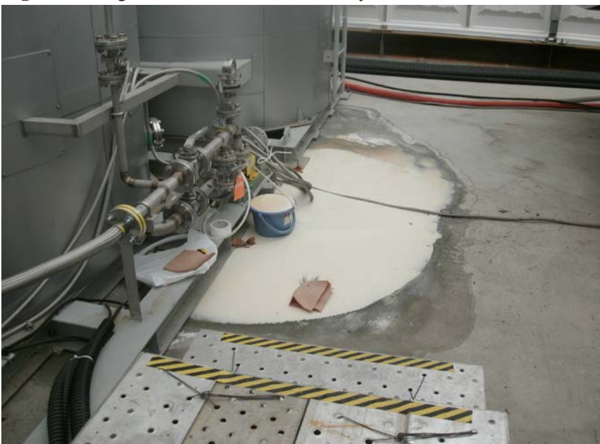
Fig 1: Leaking desalination units (Photo by TEPCO)
