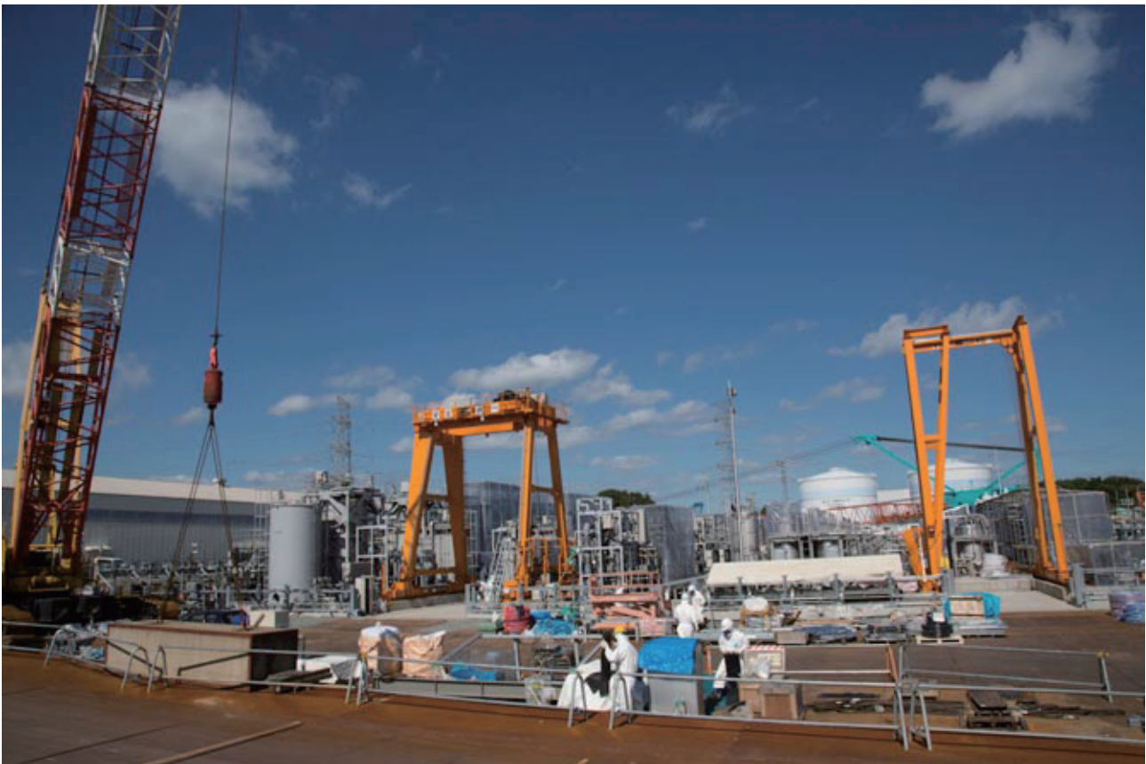
Construction of a new water processing plant 'ALPS' at the Fukushima Daiichi Nuclear Power Station, October 2012. (cc) OZAKI TAKASHI
