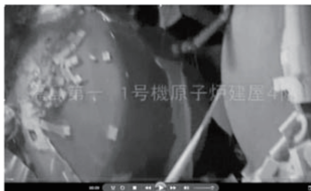
Photo 1: The two IC units (4 th fl., Unit 1 bldg.)
