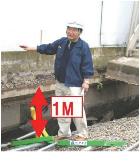
One-meter ground subsidence at KKNPS that occurred during the Niigata Chuetsu-oki Earthquake. (Reported in the 20 questions and answers on why KKNPS must not restart.)
