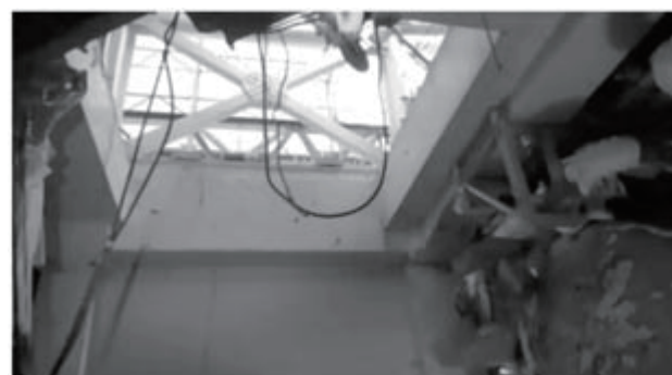
Photo 4: Looking up from the 4 th floor to the equipment hatch (the steel lid blown away by the hydrogen explosion is missing, an IC unit is visible to the right).
